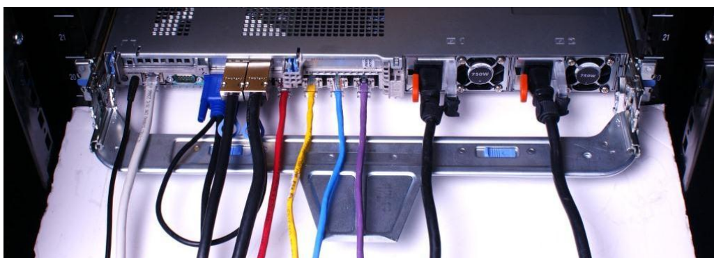
Figure 1. System with cables installed
